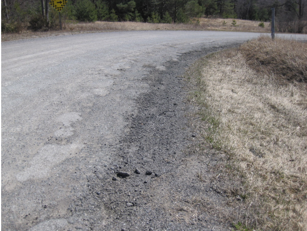
Photo 3 - Low Shoulders Inside Horizontal Curve Leading to Edge Break
