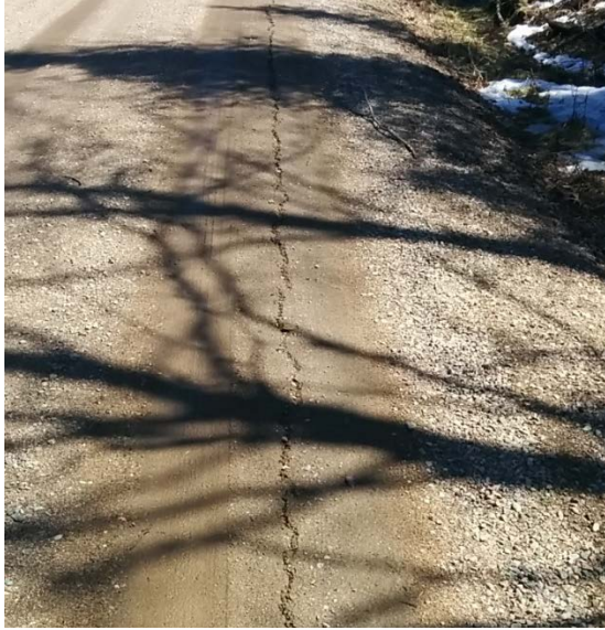
Photo 2 - Low Shoulders Against the Travelled Surface
