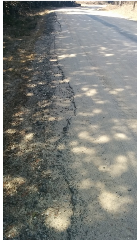
Photo 2A - Low Shoulders Leading to Edge Break
