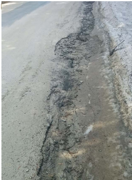
Photo 2B - Low Shoulders Leading to Edge Break
